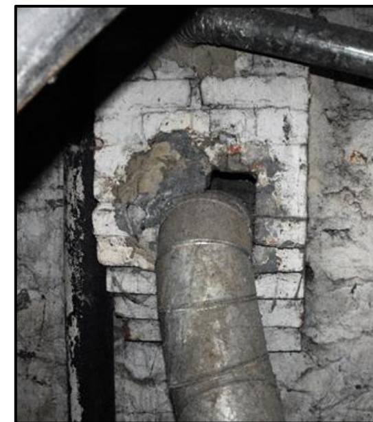
Flue not sealed to chimney
