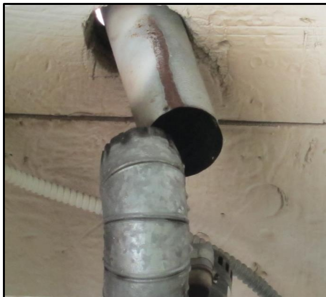
Detached sections of flue
